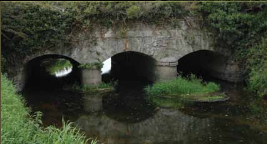
The substantial triple-arch Mountmellick Aqueduct carries the canal over the Triogue River. This was the only large river crossed by the Mountmellick Canal. To negotiate streams and drains, the Grand Canal Company constructed nine single-arch culverts, seven of which continue to function.
