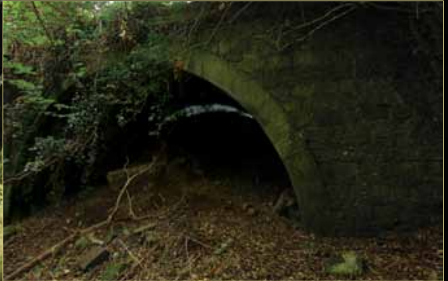
Kilnacash Bridge is one of 27 bridges built along the Mountmellick Canal. Some carried roads and railways over the canal; others carried the canal over streams and drains. Today 23 of the original bridges continue to function.
